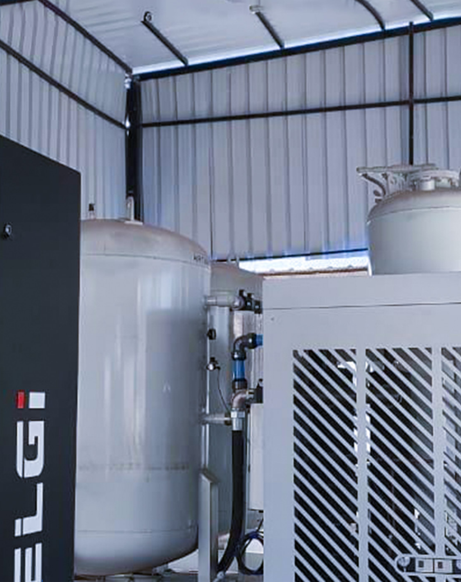
View of a PSA Medical Oxygen Generation Plant set up by RAF Global and Zarina Foundation at GMERS General Hospital, Junagadh (Gujarat) India, 2021
